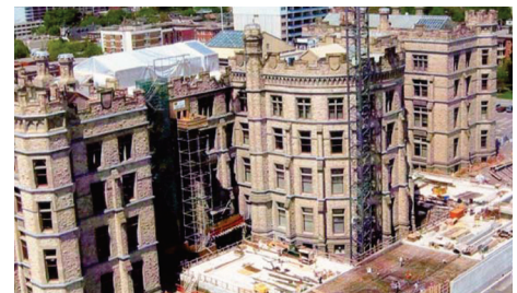
VICTORIA MEMORIAL MUSEUM OF NATURE, DEMOLITION, ASBESTOS REMOVAL AND MOLD REMEDIATION OTTAWA, ONTARIO
